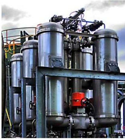
Biodiesel Crossflow Filtration System
