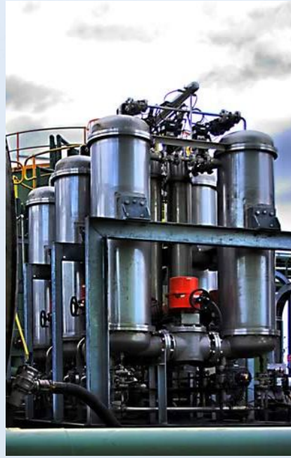
Industrial Crossflow Filtration System
